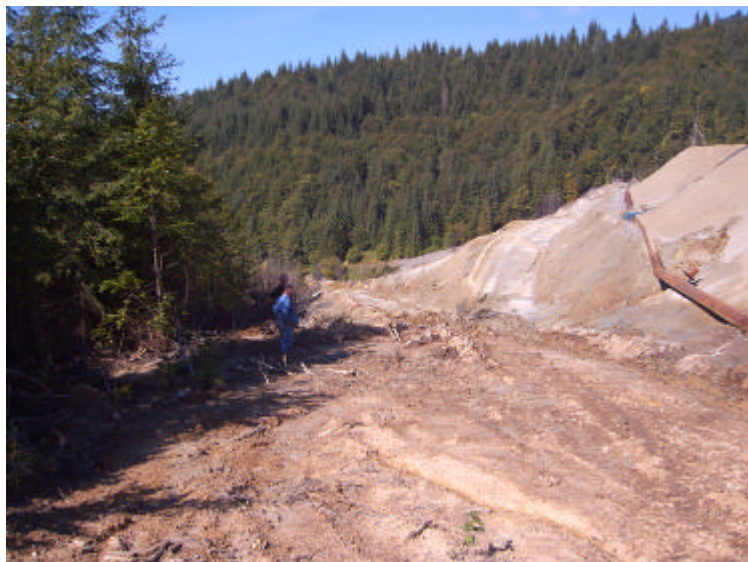
Two new access roads were built during the rehabilitation project to more easily reach the main units of the tailings pond, here the access from the top to the bottom (toe) of the main dam (photo: Horvath).
