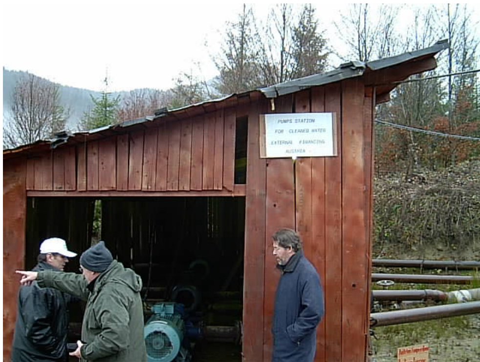
The repaired pumping station for cleaned water (main tailings pond): Mr Mois (REMIN envir. dep., Prof. Lorber/AT and Mr Zinke/AT).
