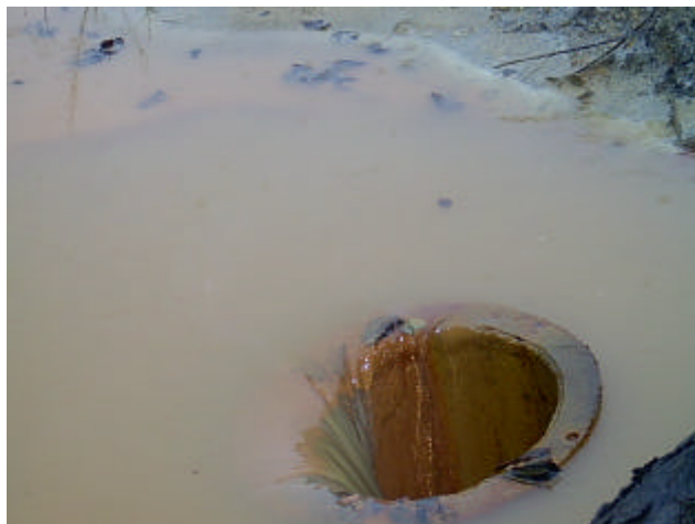
Penstock at the lowest point of the exfiltration pond (photo on top): From here seepage water is designed to go through the pipe via the exfiltration pond pumping station back up to the main pond (closed circuit).
