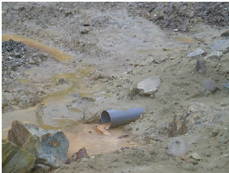
Detail from the toe of the main dam: As a result of the new drainage system, pipes collect seepage and spring water in a controlled way and discharge it downstream to the exfiltration pond.
