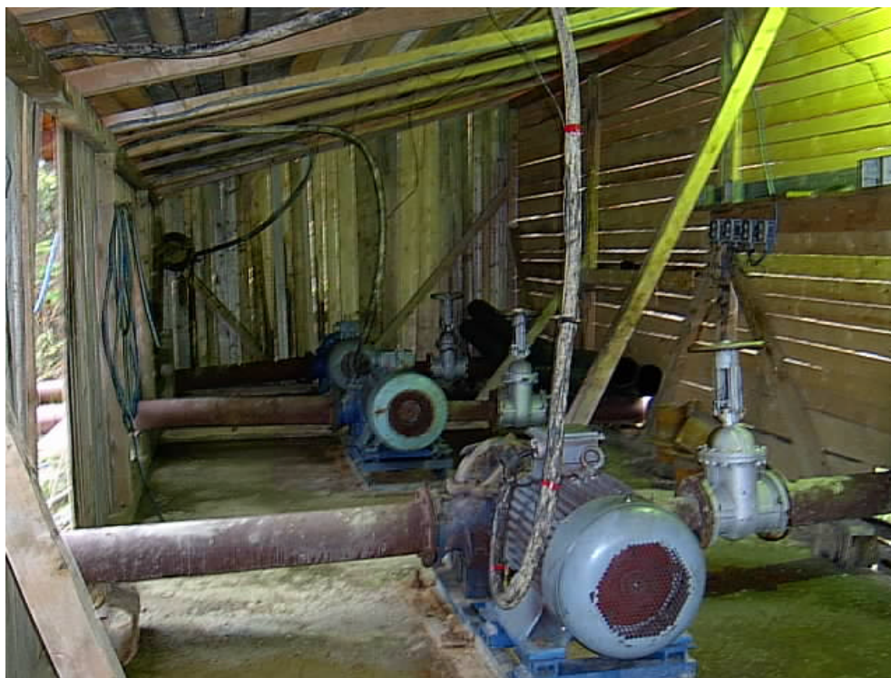
The new pumps at the repaired pumping station of the main tailings pond
