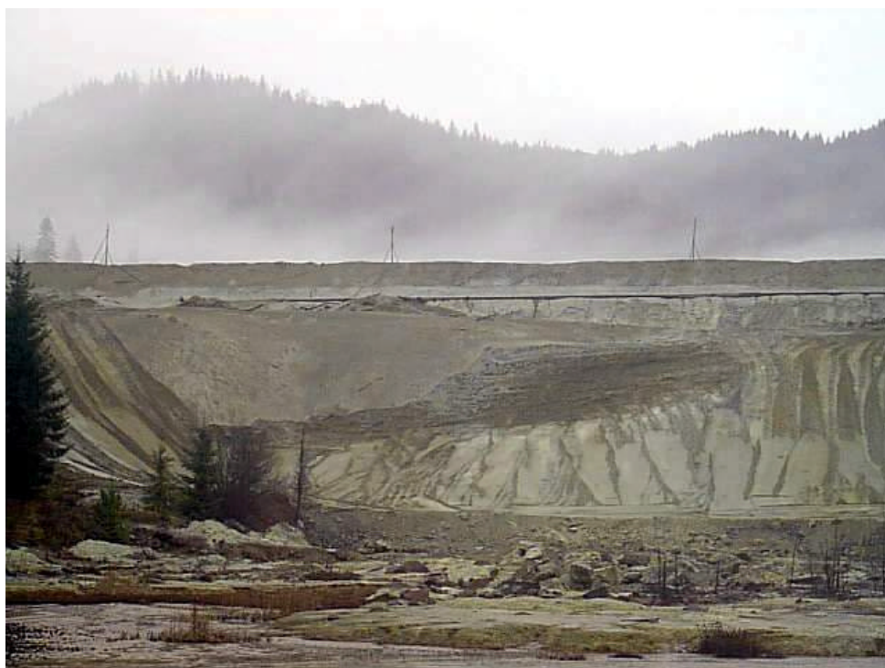
View from the exfiltration pond upstream to the rehabilitated (more gentle) slope of the tailings dam. Below the pipeline the intermediate berm can be seen; at the toe a new drainage system was built in. (photo: Stematiu)
